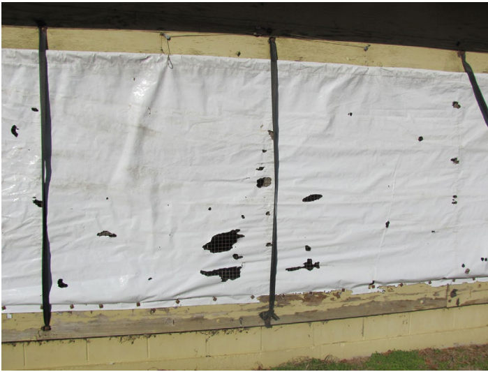
Figure 1. Rodent damage may start small.
