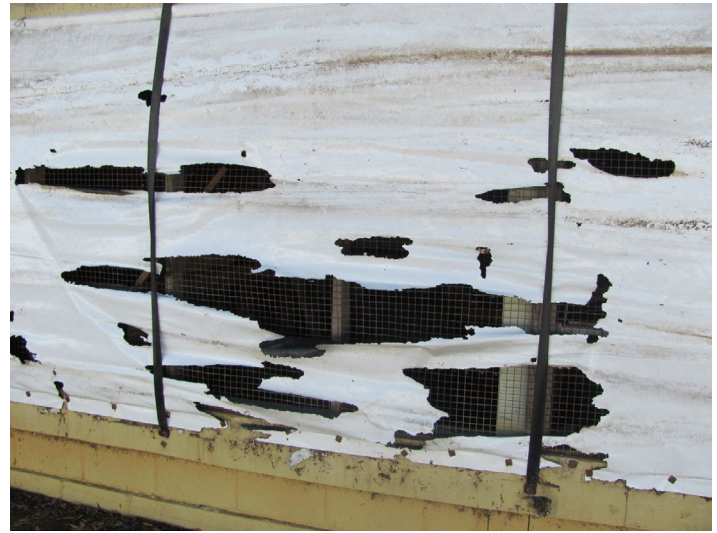
Figure 2. Damage can quickly escalate into a major problem.
