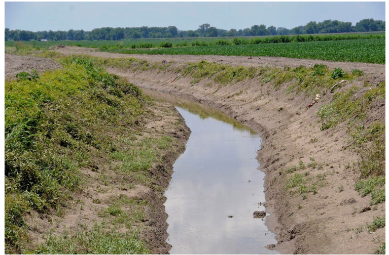
Figure 11. A drainage ditch that has undergone construction to widen the channel and create floodplain benches to create a two-stage ditch.
