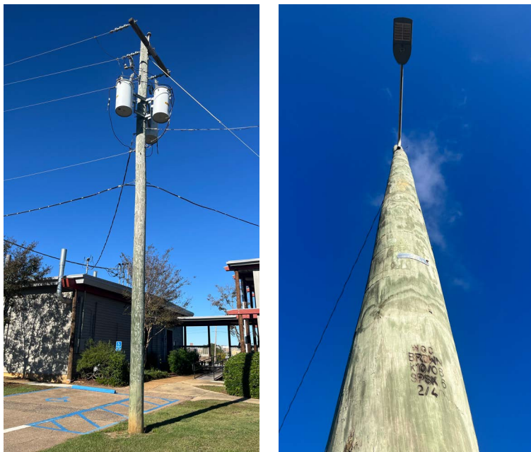
Figure 13. Wood utility poles.
