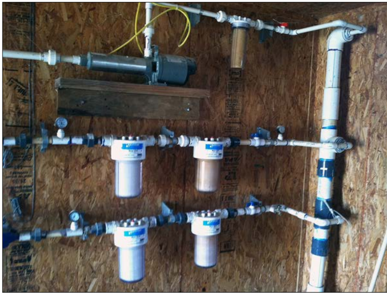
Figure 3. A 4-inch supply line from the well with 1-inch distribution lines to the drinkers in the front and back halves of the house and to the cooling system.
