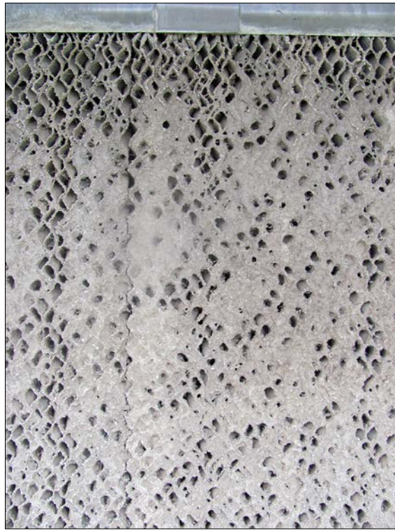
Figure 1. Cool cell pads clogged by mineral deposits.
