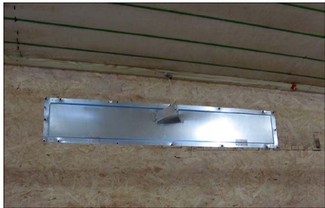
Figure 5. Sidewall air inlet.
