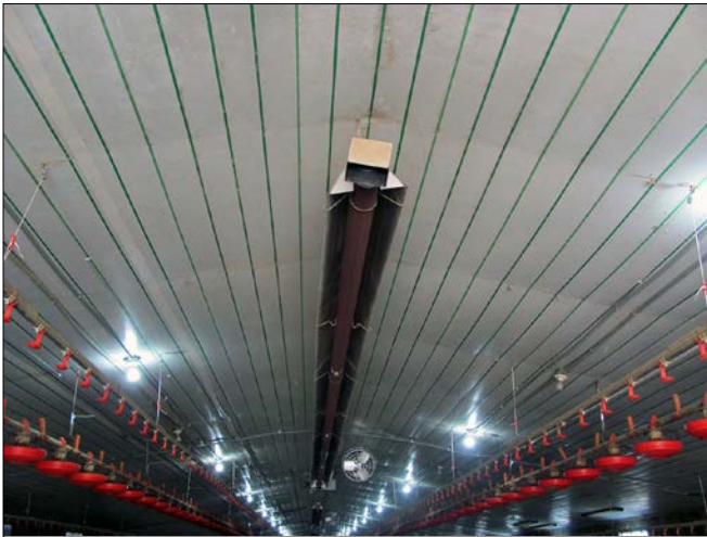
Figure 2. Tube heater in a broiler house.
