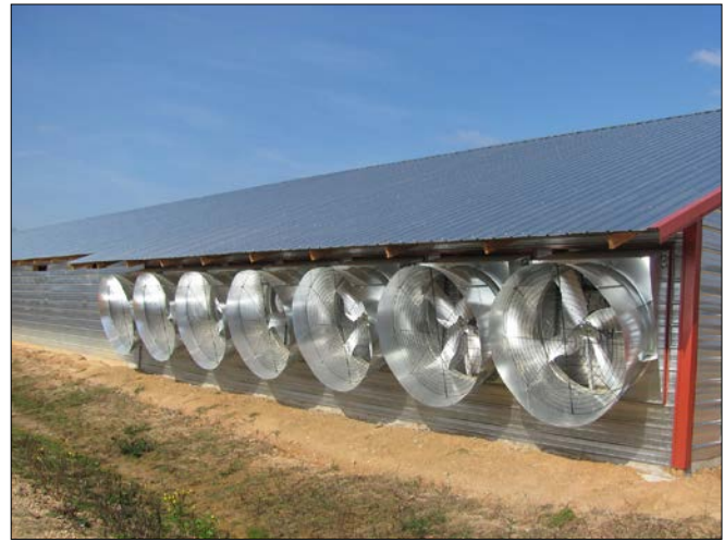
Figure 4. Fans in a broiler house.
