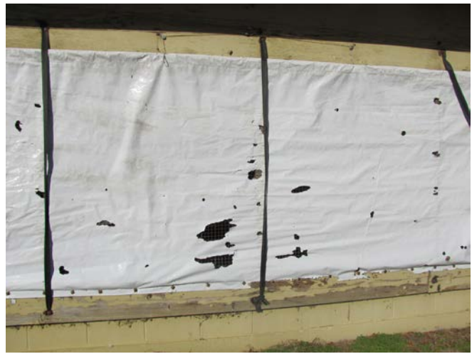
Figure 1. Rodent damage may start small.
