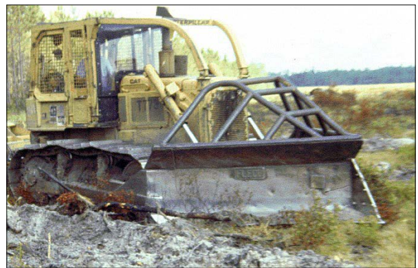
Figure 2. Land-clearing involves shearing large material with a tractor-mounted blade or chain saw.
