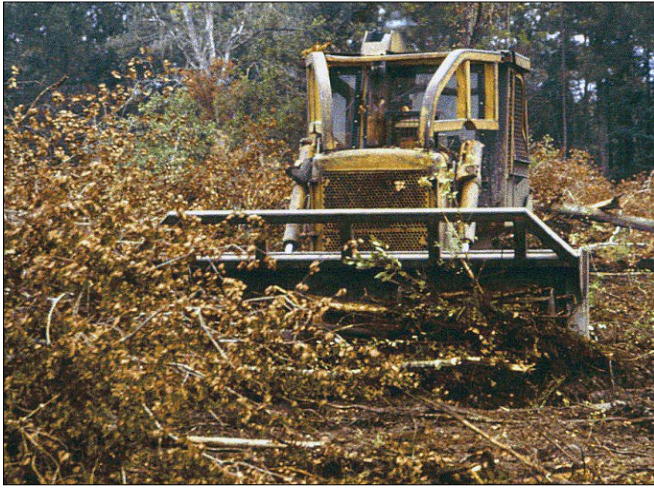
Figure 3. Once felled, debris is raked into piles or rows to complete the land-clearing operation.
