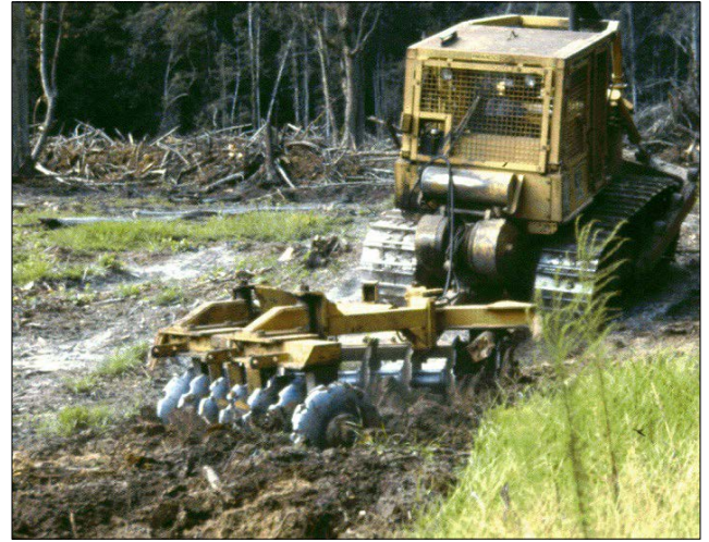
Figure 5. Disking with an offset harrow controls competing vegetation by cutting and exposing roots. Disking can also restore the site from rutting and compaction during logging and land-clearing.
