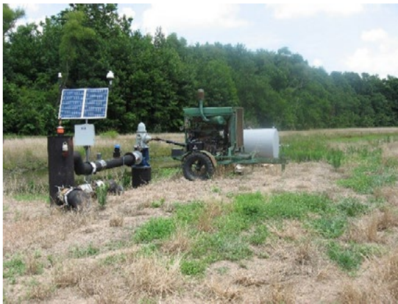
Figure 5. Pump to move water from tailwater recovery ditch to OFS.
