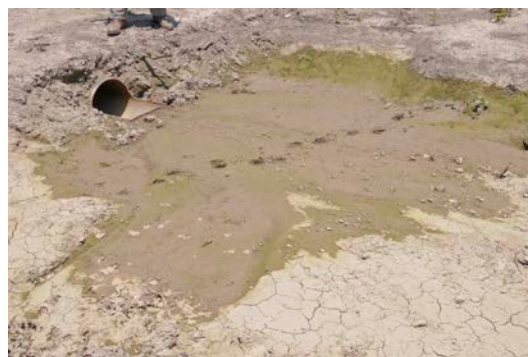
Slotted inlet pipe beneath levee for grade stabilization and erosion control in the Mississippi Delta. Photo credit: REACH program
