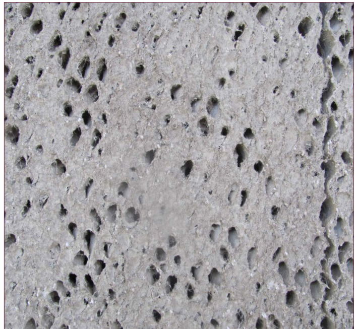
Figure 3. Mineral buildup clogs cool cell pads.
