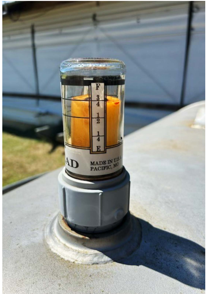
Figure 5. Sight gauge for backup generator fuel tank.
